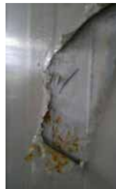
Example of oxidation after blistering
